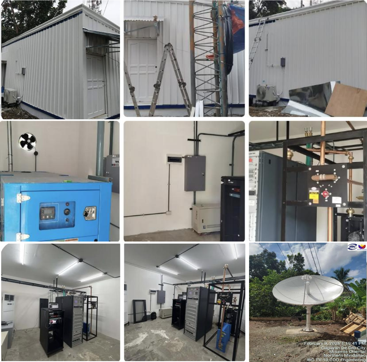
NEW CDO SITE, TRANSMITTER TOWER, TVRO SYSTEM
