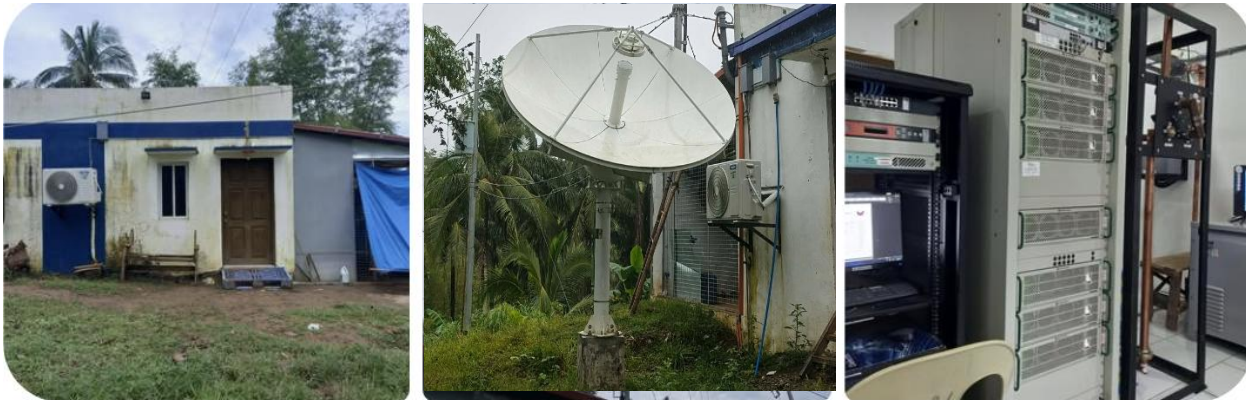
SITE LOCATION WITH GENERATOR
