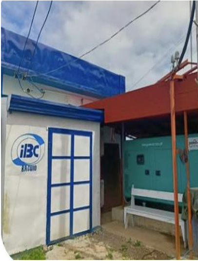
SITE LOCATION WITH GENERATOR
