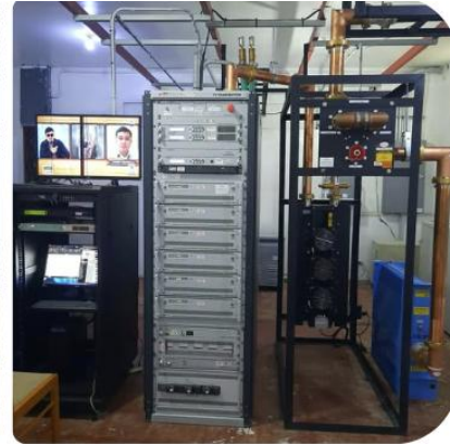
NEW DTT TRANSMITTER
